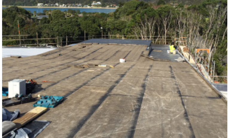
RL Derbicoat Base Sheet installed over RL Roof Board HD for the Waitangi Museum project.
